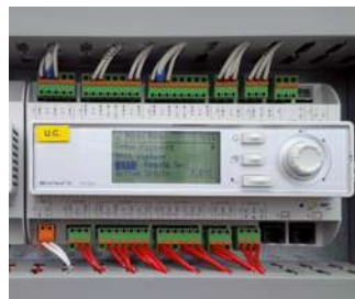
Controller box upgrade
